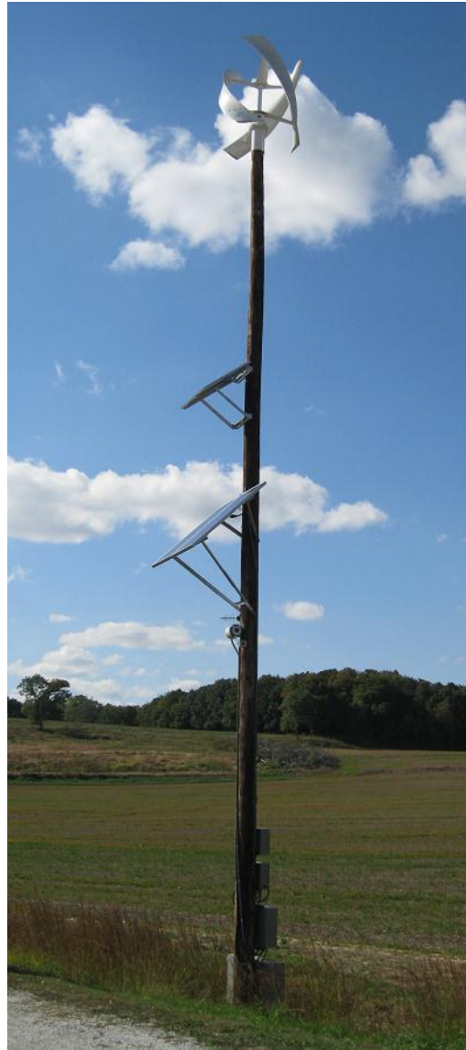
Figure 67: Upgraded Renewable Energy System
