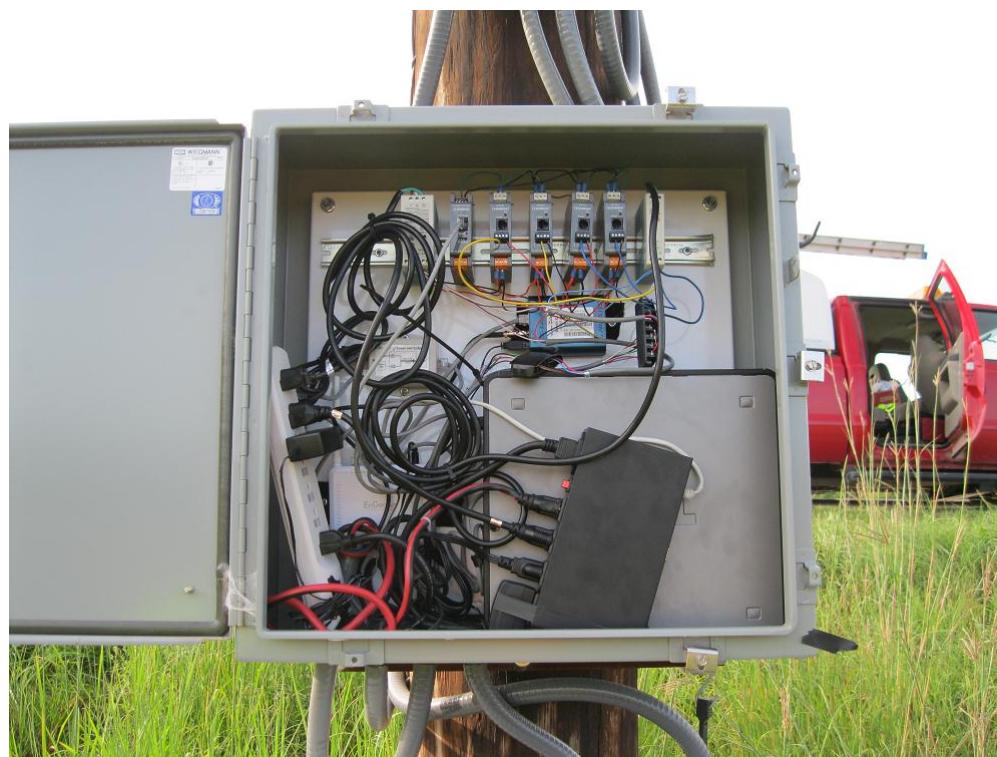
Figure 62: Inside of Typical NEMA Enclosure
