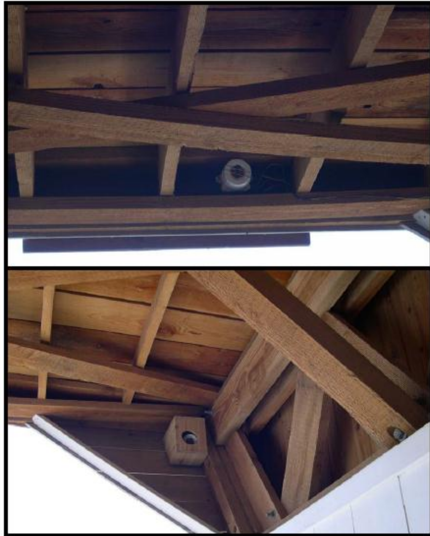
Figure 64: Flame Detectors with and without Wood Coverings
