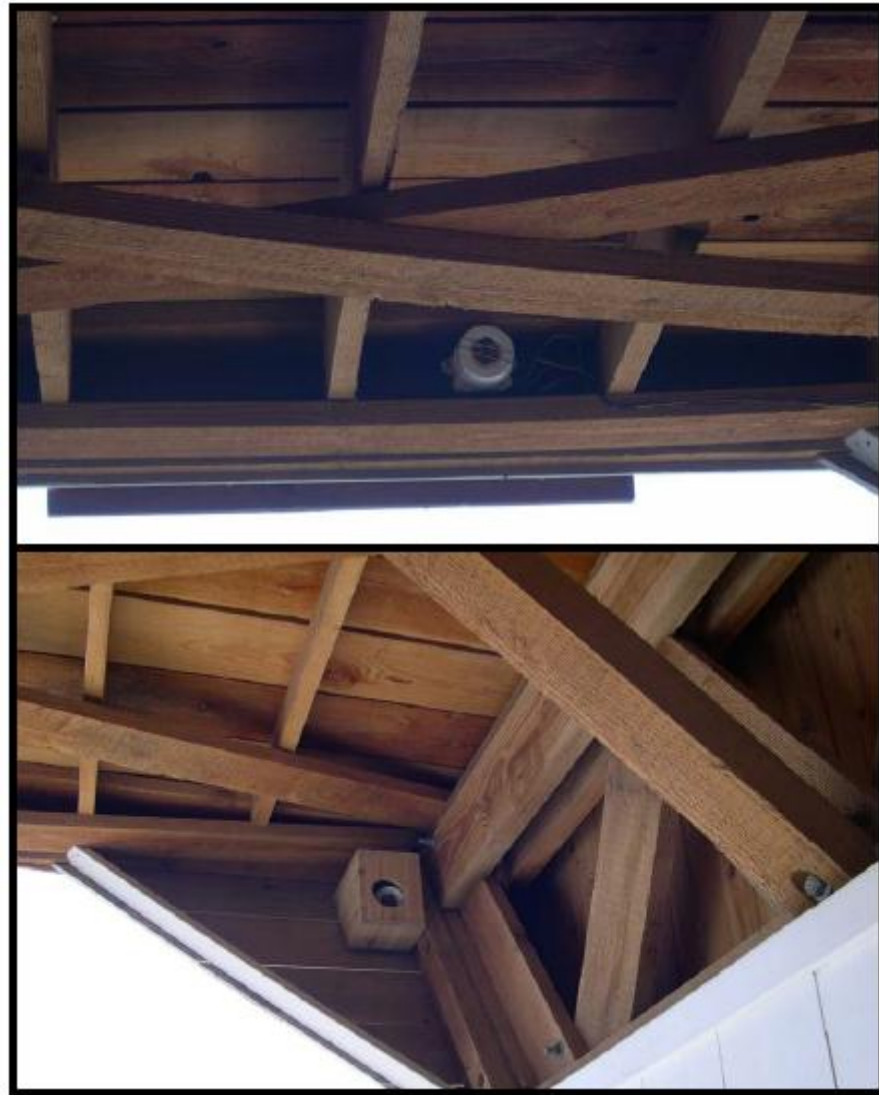
Figure 9: Flame Detector in Covered Bridge without Encasement (top) and With Encasement (Bottom)
