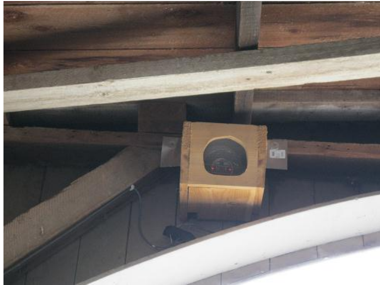
Figure 71: Flame Detector after Alarm Set Off
