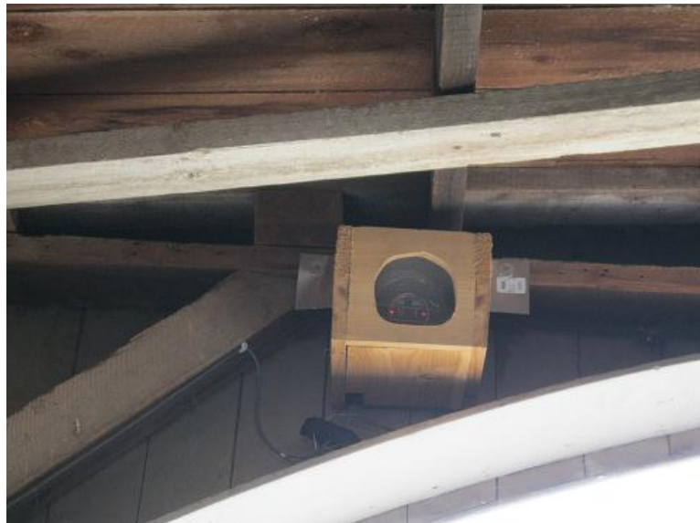
Figure 55: Flame Detector after Alarm Set Off
